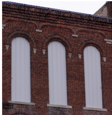
Inappropriate upper windows
